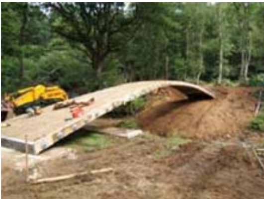
The new bridge at Hawnby under construction - it was installed as part of the flood recovery programme.
