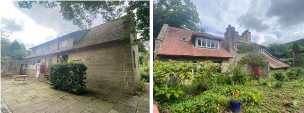
Front and rear elevations of the first floor lona flat above the stables
