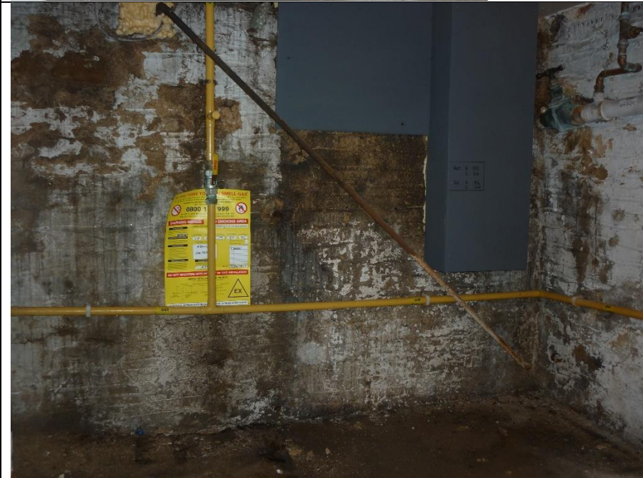
Entire basement was wet.
