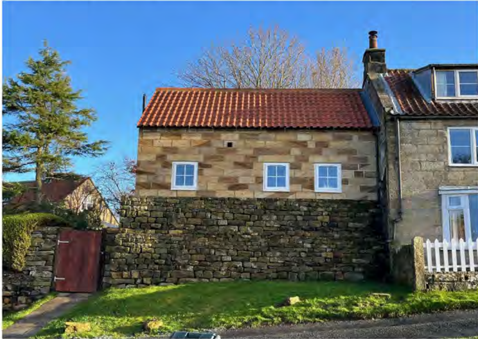
Fig 1E: Photograph of the constructed extension. The drystone wall has been photoshopped to appear complete. Completion of the stone wall will hopefully take place shortly. This week weather permitting.
