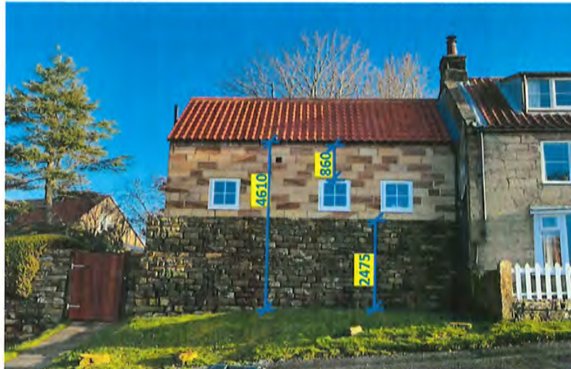
Fig 2: As-built extension – Smaller than the approved design. It is built from the same approved wall and roof materials. (Drystone wall photoshopped to appear complete. Completion on site will hopefully be this coming week).
