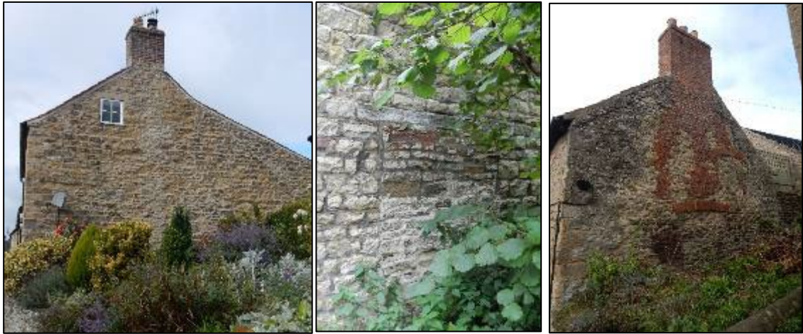
Figure 35, 36 & 37: Blocked openings in the kitchen garden wall show where hot houses were located; the gable ends of houses show evidence of former buildings, increased, or altered roof lines and rebuilt chimney stacks (often after a fire). Fields to the rear of the
