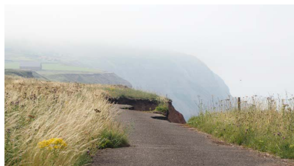
Fig.144 Coastal road lost to a landslip north of Staithes. Boulby Head is shrouded in mist in the distance.
