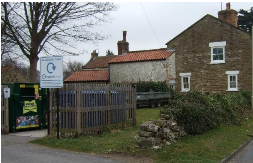
Photo 38: Collapsed section of stone boundary wall
