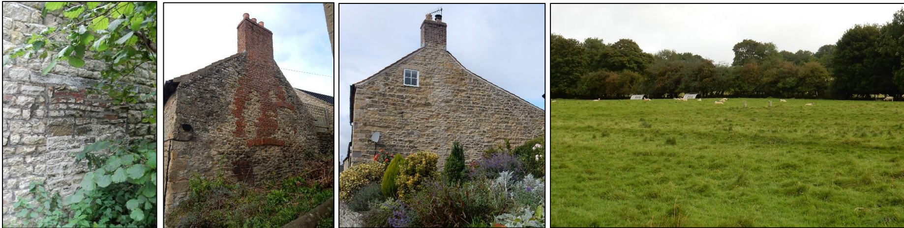
Plate 12. Blocked openings in the kitchen garden wall show where hot houses were located; the gable ends of houses show evidence of former buildings, increased or altered roof lines and rebuilt chimney stacks (often after a fire). Fields to the rear of the houses often contain evidence of ridge and furrow showing where centuries of ploughing have taken place.
