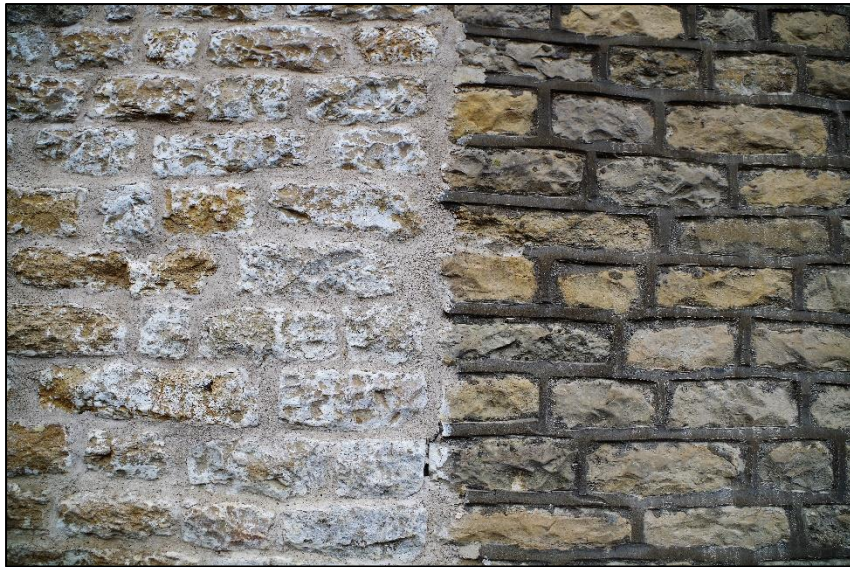
Plate 16. Different ownership has resulted in different approaches to pointing. The ribbon pointing on the right will damage the stonework over time.
