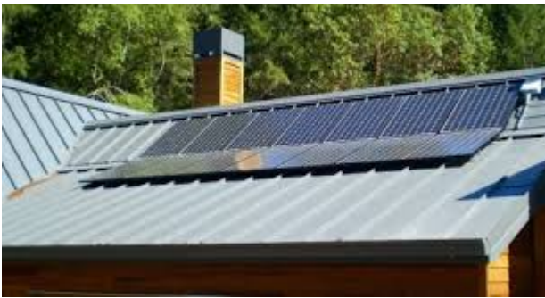
Figure 5.1 Photovoltaic cells on a standing seam roof
