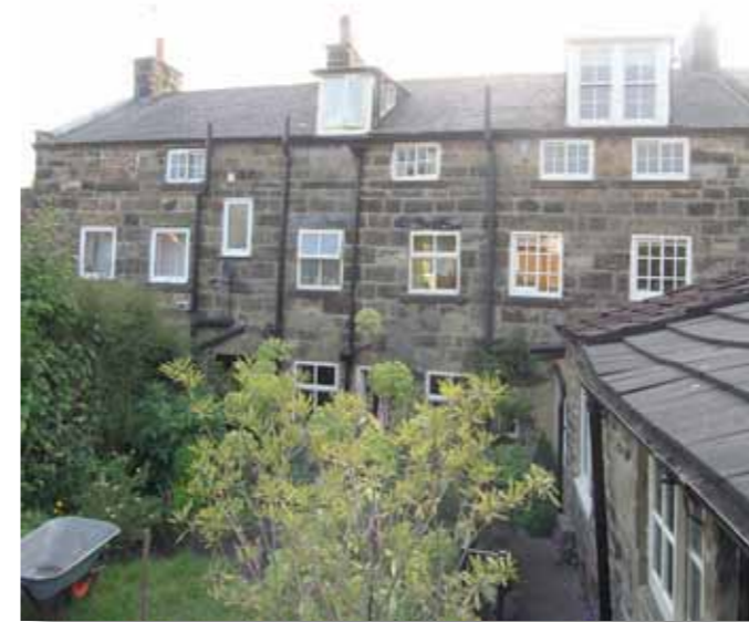
Above: Weavers terrace in North End with communal workshop in the attic, which would have been poorly lit by the shallow top windows before the recent dormers. Note the missing window preserved in the adjacent out-house.
