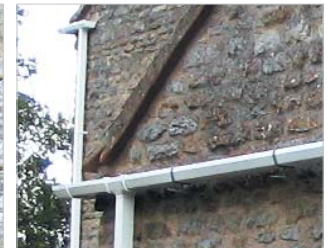
Avoid square section and/or white rainwater goods
