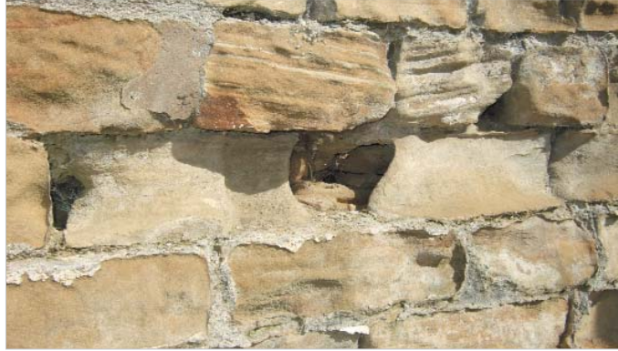
Erosion of the weaker stone
