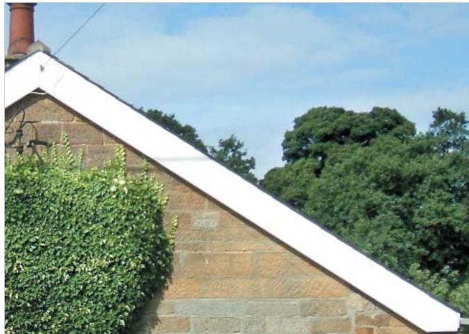
Inappropriate barge board
