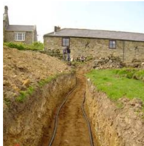
Installing ground source heat pumps can cause significant earth disturbance which should be restored.
