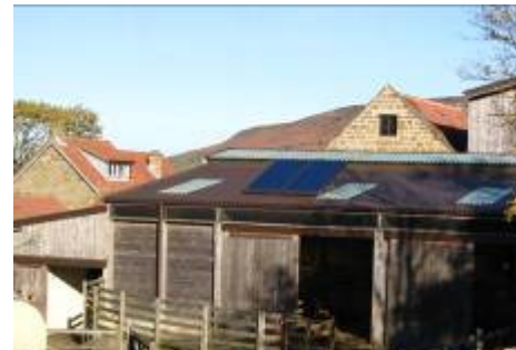
Solar panels can be well suited to industrial or agricultural style buildings
